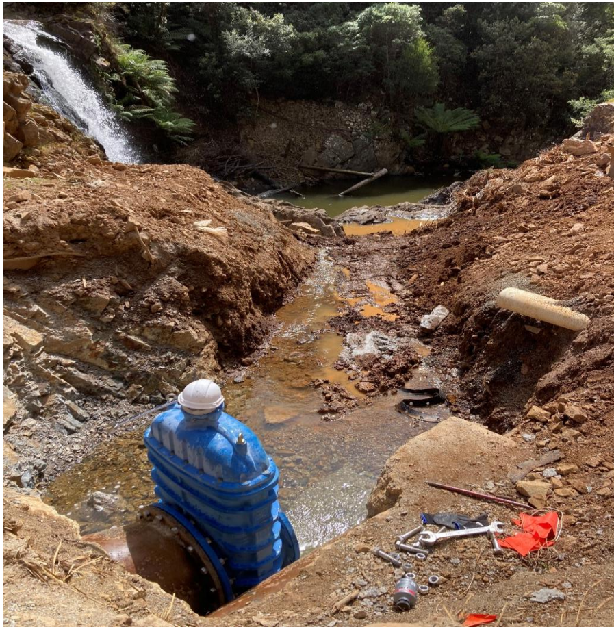
Figure 12 New Scour Isolation valve Isandula Dam
